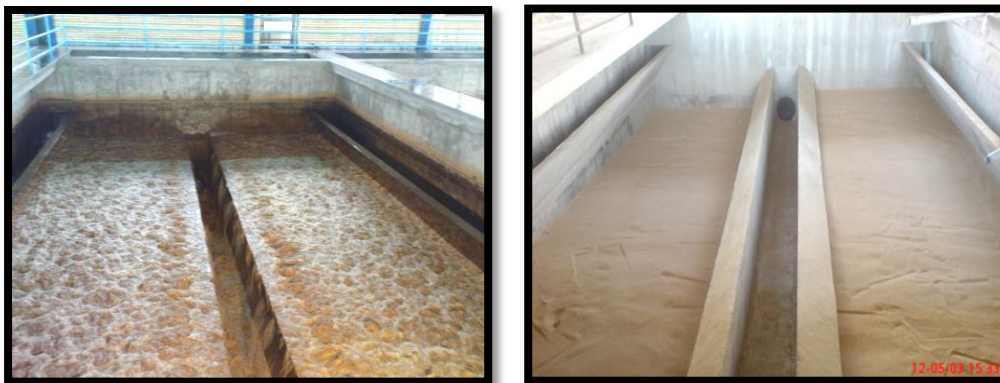
Fig. 2. The view of Rapid Sand Filter bed.
