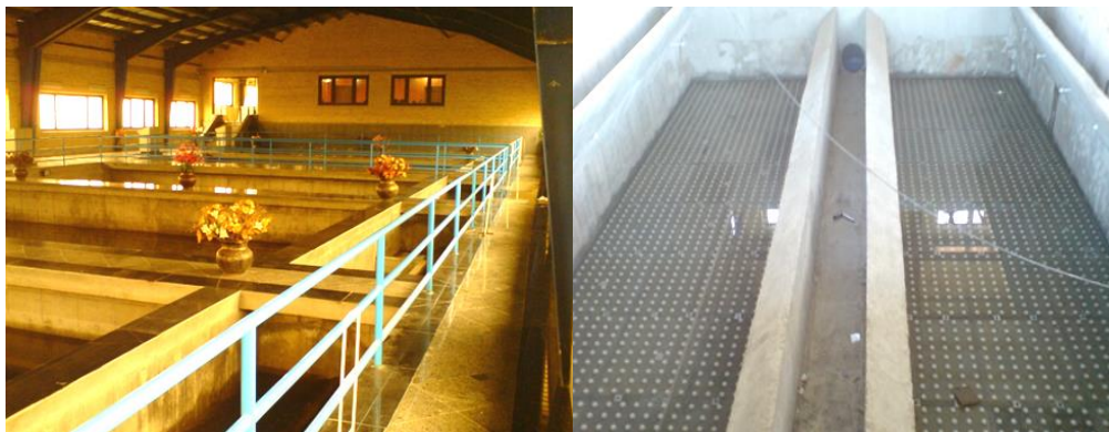
Fig. 1. The view of filtration hall and sand filter bed.
